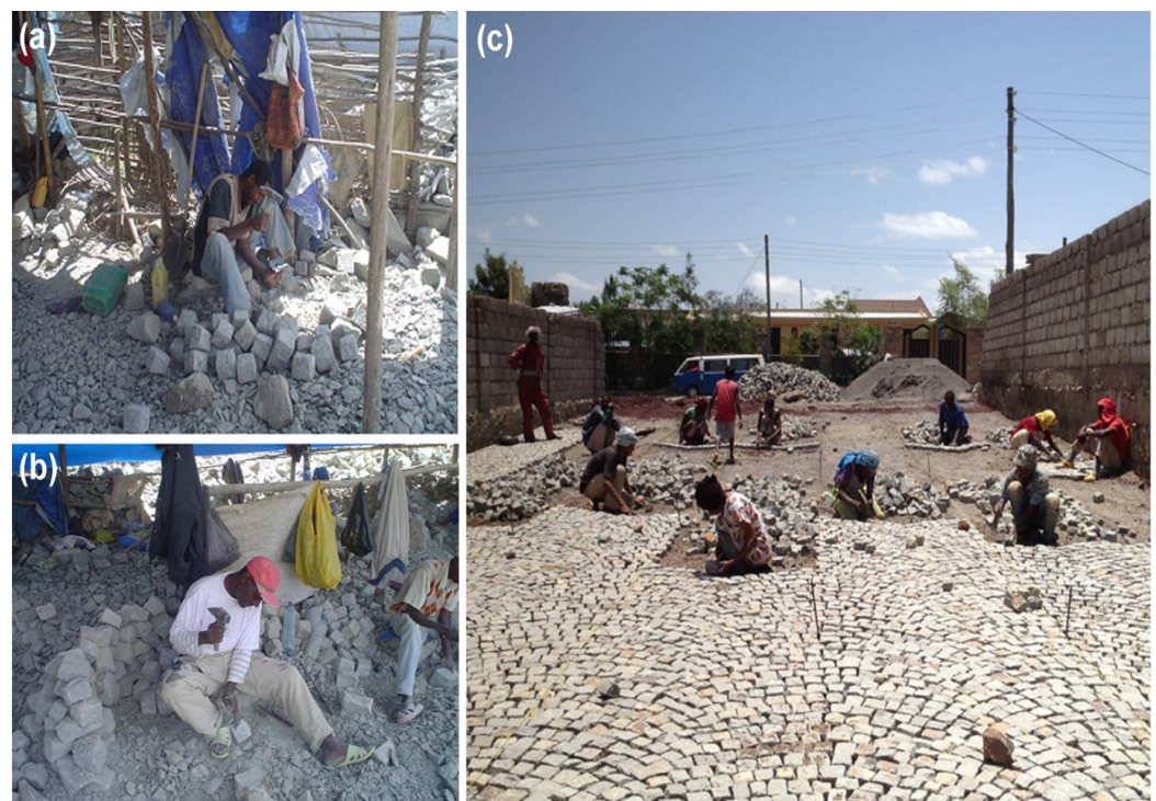
Figure 2. Cobblestone works: (a) chiseling site 1, (b) chiseling site 2, and (c) road paving.
