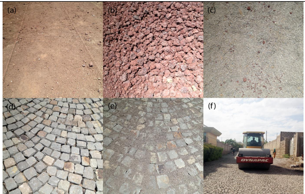
Figure 1. Construction of cobblestone road in Adama, Ethiopia: (a) the leveling of a road, (b) red lavas, (c) crushed sands, (d) cobble stones, (e) fill the gap with crushed sands, and (f) complete leveling of road using a roller.
